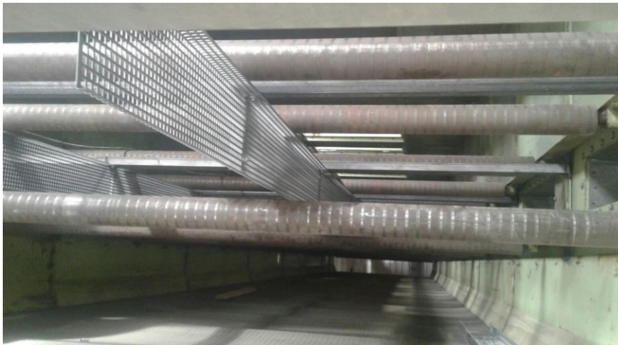
Fig. 5.3: Drying belt with diffusor plates installed and air intakes on the right hand side
