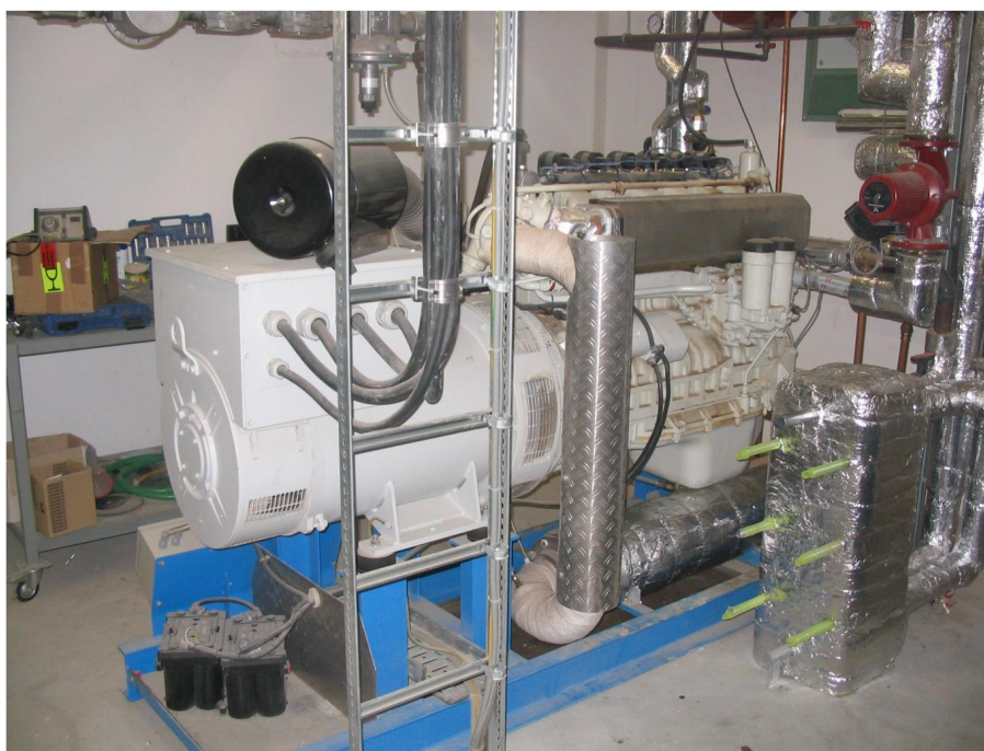
Abb. 4: 190 kW el. Gas-BHKW in der Praxis
