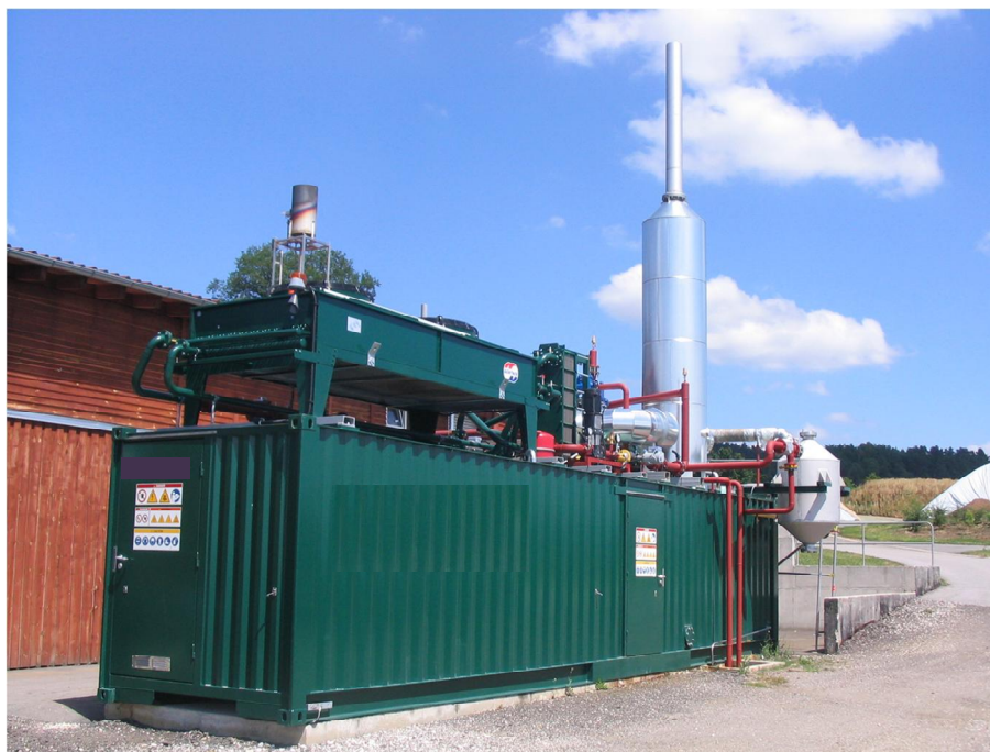
Abb. 7: 526 kW el. Gas-BHKW in der Praxis
