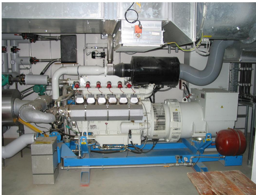
Abb. 6: 324 kW el. Gas-BHKW in der Praxis
