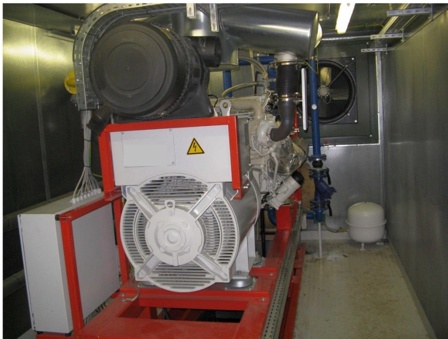
Abb. 5: 250 kW el. Gas-BHKW in der Praxis
