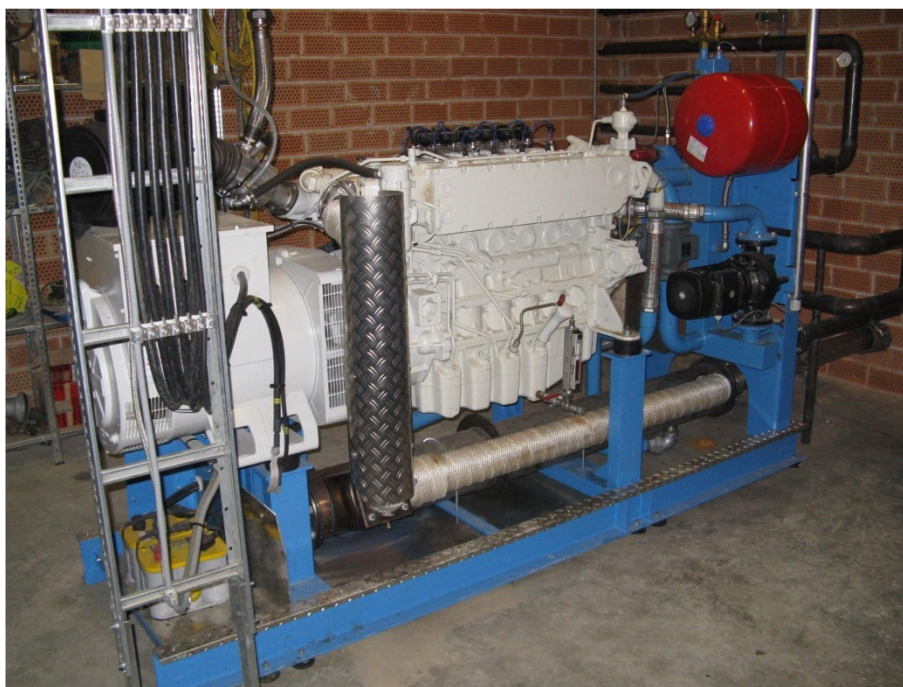
Abb. 3: 100 kW el. Gas-BHKW in der Praxis
