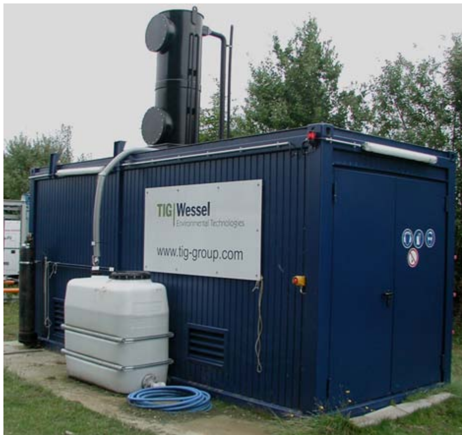
Fig. 6: Pilot plant in Albersdorf, Schleswig-Holstein
